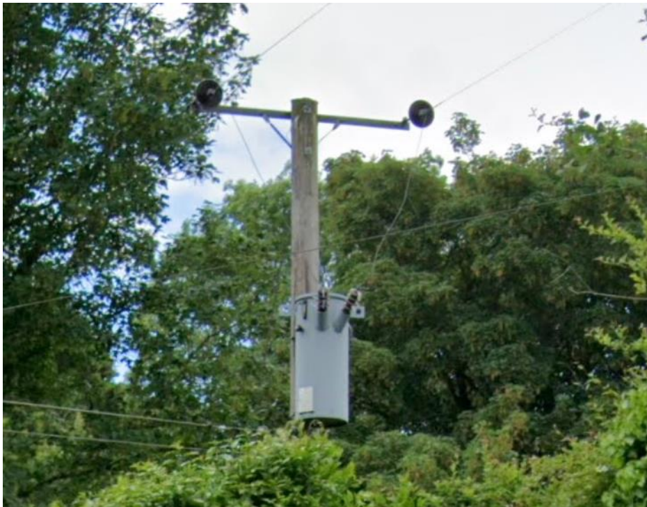
Figure 27 Duxmoor pole-mounted transformer, showing split-phase HV connection 40 where the HV circuit only has two phases
