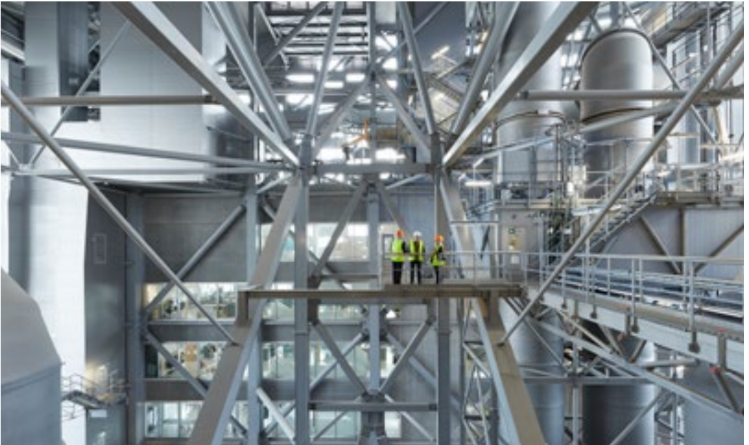
Inside Copenhill, modern waste treatment machinery is all arranged in height order, which forms the building’s sloped rooftop and resulting 9,000-metre-squared ski and recreational terrain. Photograph by Soren Aagaard
